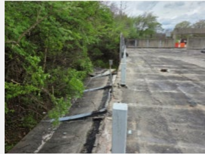
Area of wall failure
