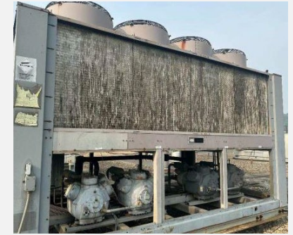
Roof Mounted Chiller
